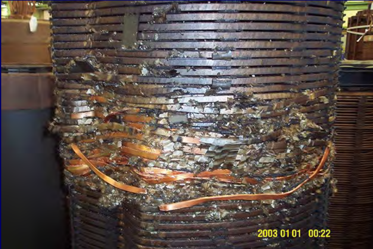
Power Transformer Winding Damage
